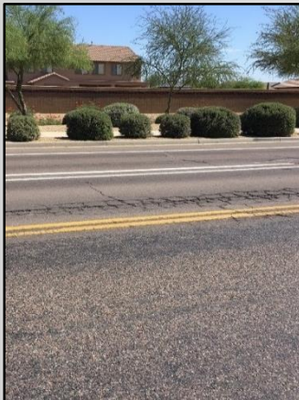
Before Rehab Example (Cracking in Peoria Ave)
