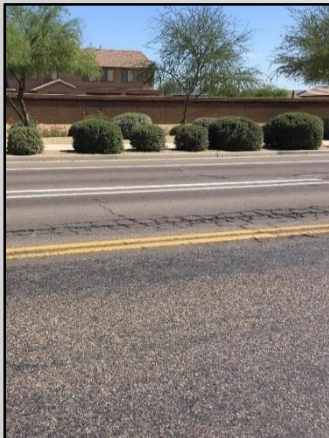
Before Rehab Example (Cracking in Peoria Ave)
