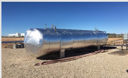
Additional Thermal Storage
