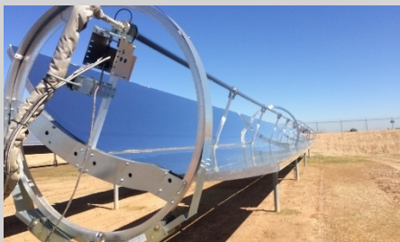
Additional Solar Collectors
