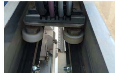
Energy Chain connection to Dryer
