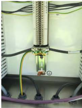
Junction Box Termination of Energy Chain prior to the energy chain
