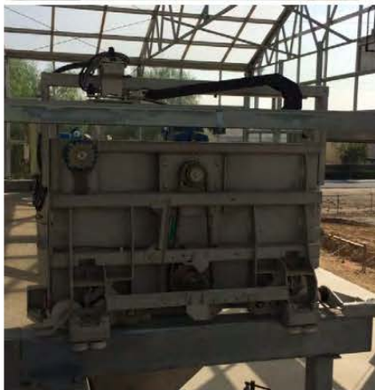
Energy Chain connection to Dryer – after the energy chain
